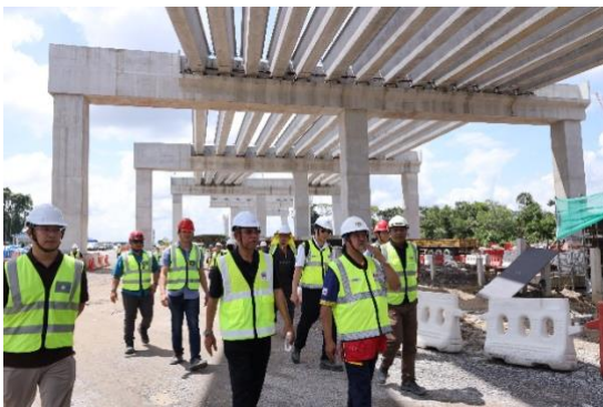
Bahrudin (2 nd right) touring the SR10 ART Interchange station (Simpang Tiga) construction site
